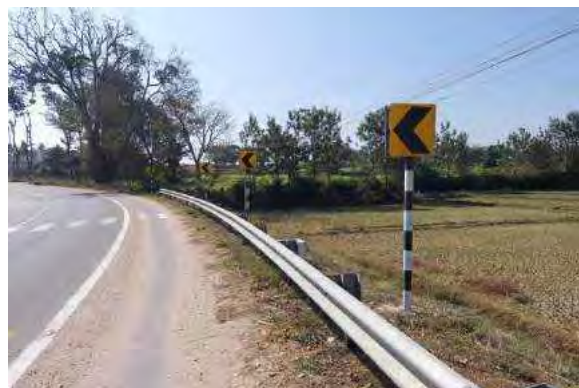
MBCB & Chevron signs in link-B
