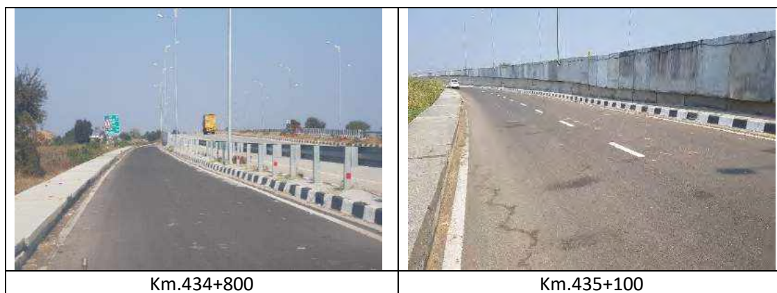
Figure 3-2: Representative Photos of Pavement Condition.
