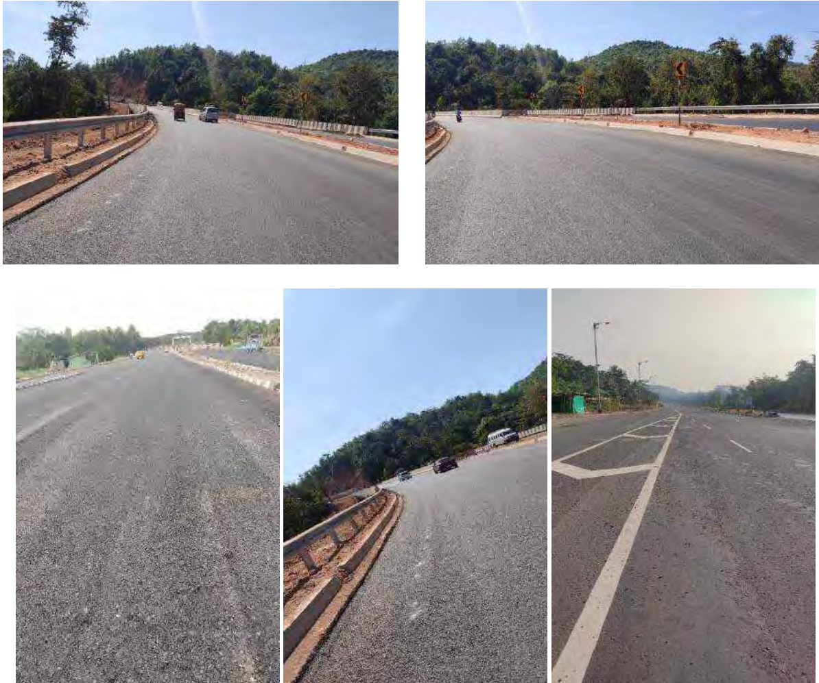
Figure 3.1: Representative Photos of Pavement Condition.
