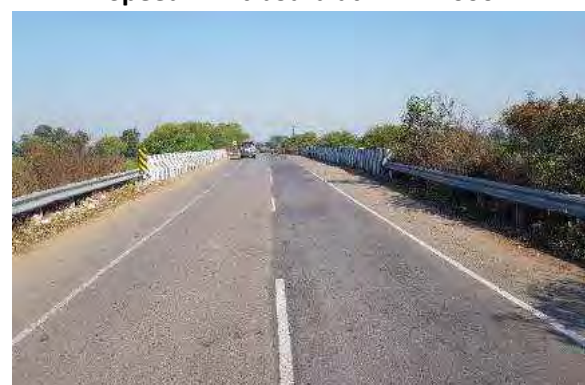
Safety at bridge approaches at Km. 4+250
