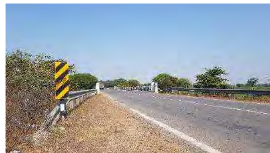
OH marker board before the Head wall of Box MJB at km.41+600
