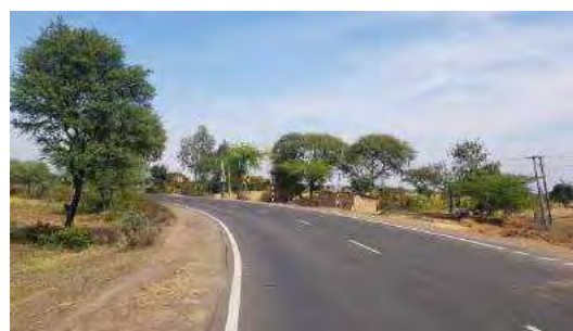
Km. 4+00 Chevron signs on the curve section
